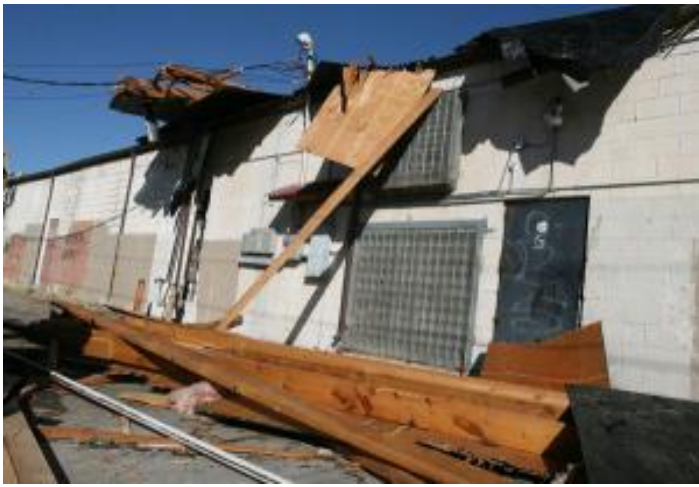
Wind gusts around 50 mph damaged this building in El Paso on October 25. (Victor Calzada /El Paso Times)
