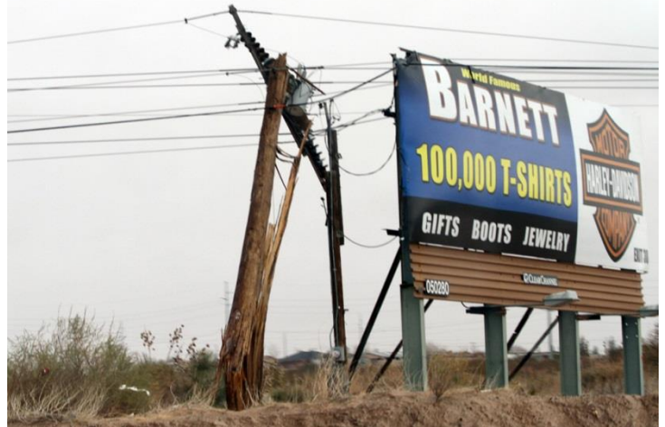
Strong winds damage this El Paso power line on December 14. (Vanessa Monsisvais El Paso Times)
