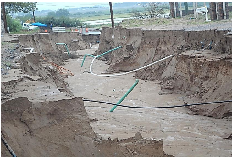
Heavy rains severely damaged La Union NM on September 12. (John Fausett NWS)
