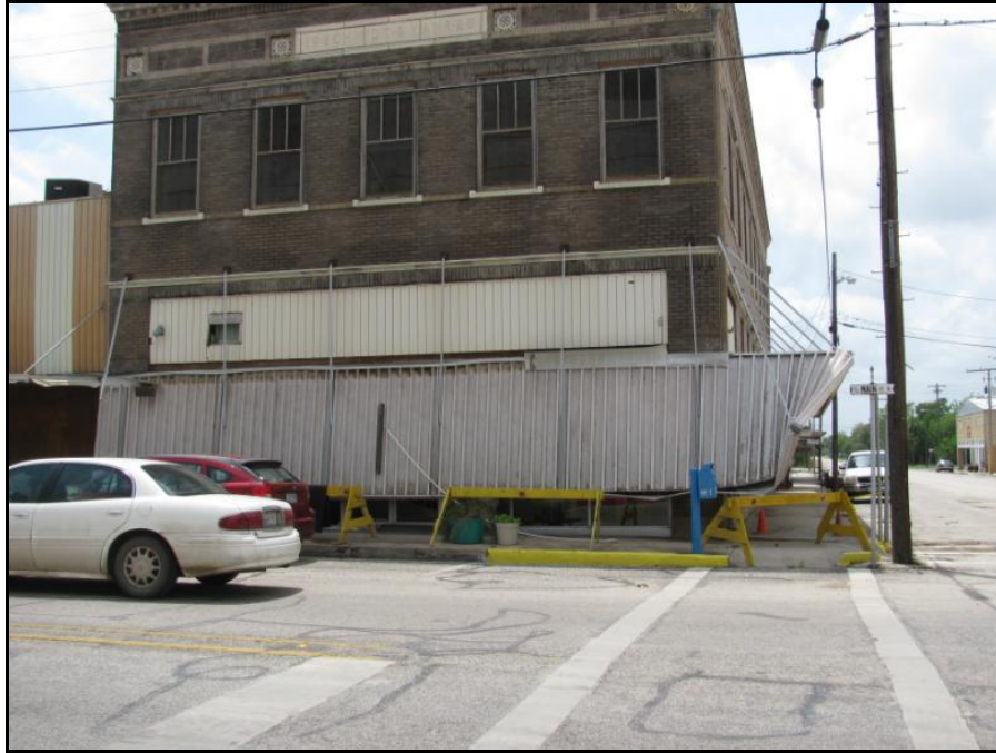
Metal awning damaged at Main and Riedel streets in Yorktown, TX
