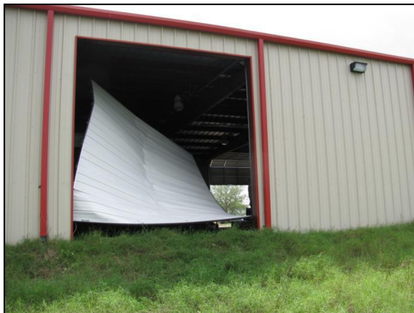
Metal building door damaged near FM 953 and Wofford Lane
