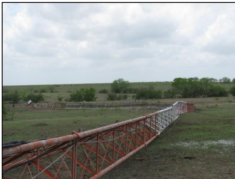
Toppled 354-foot communications tower near Muschalek Road
