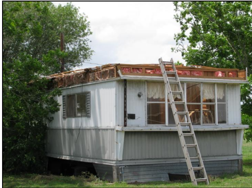
Damage to the mobile home on VFW Road
