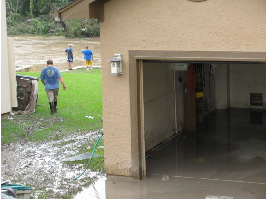
Photo 13, Water damage on the banks of the river
