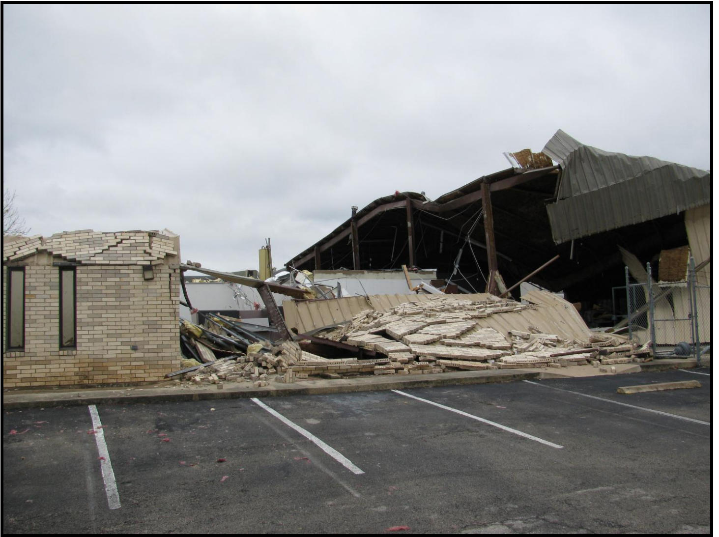
Figure 6. Damage to an industrial building on Commercial Park Drive in northeast Austin.
