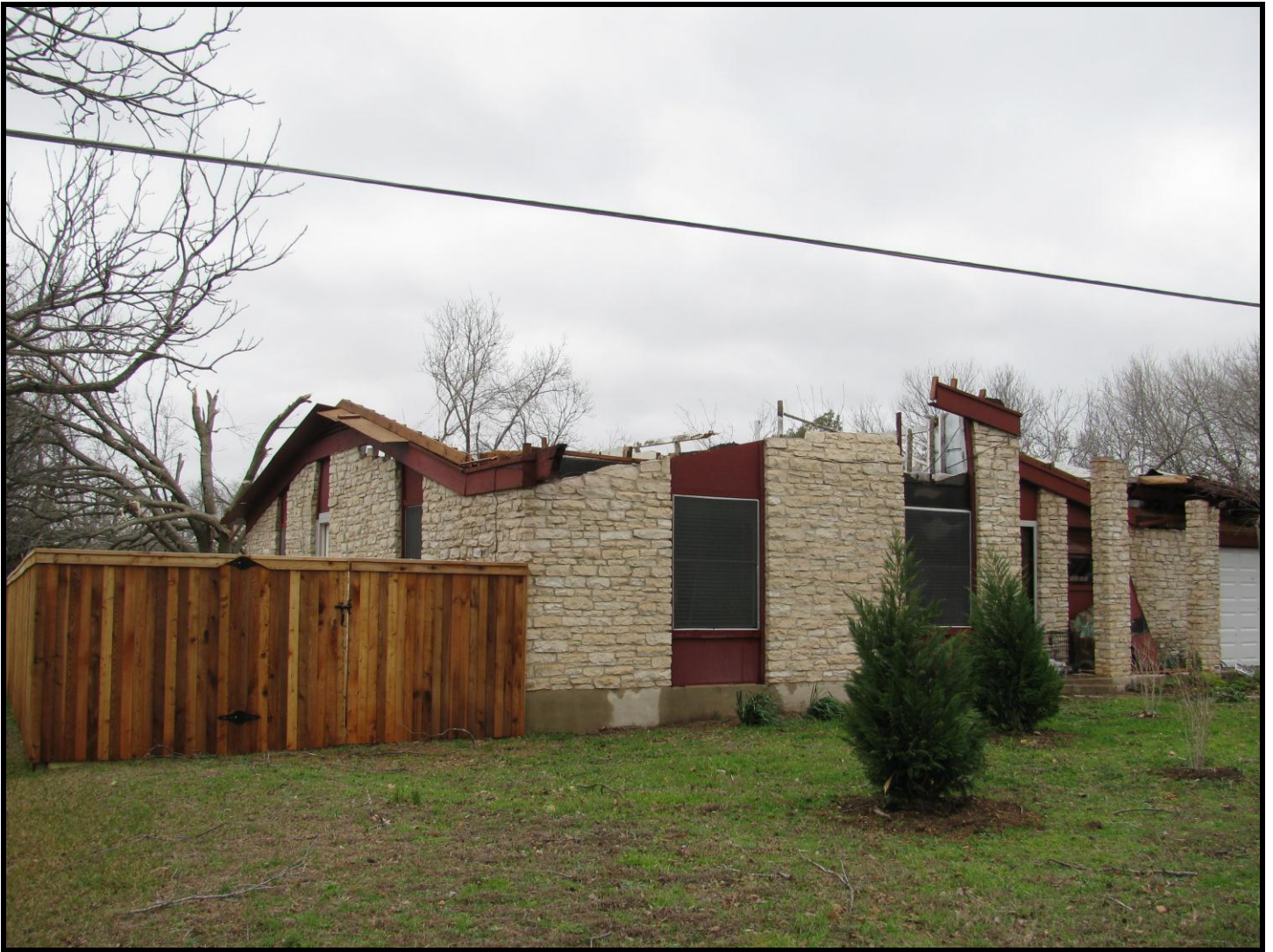
Figure 5. The roof was taken off this home on Happy Trail in northeast Austin.
