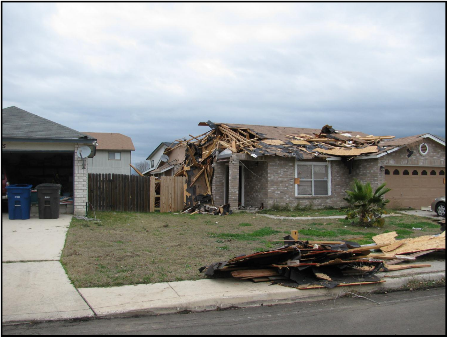
Figure 8. Extensive roof damage to a home on Deer Park in southwest San Antonio.
