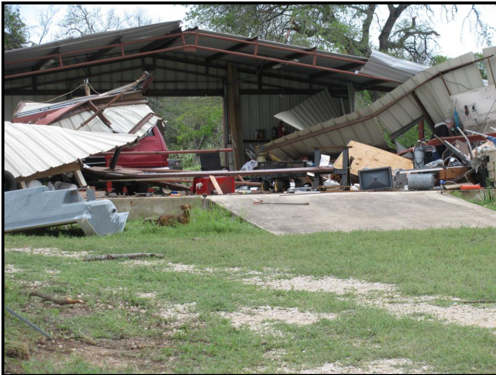
Figure 5. A steel frame shed severely damaged by the EF1 Tornado near Natalia, TX, on March 19, 2012.
