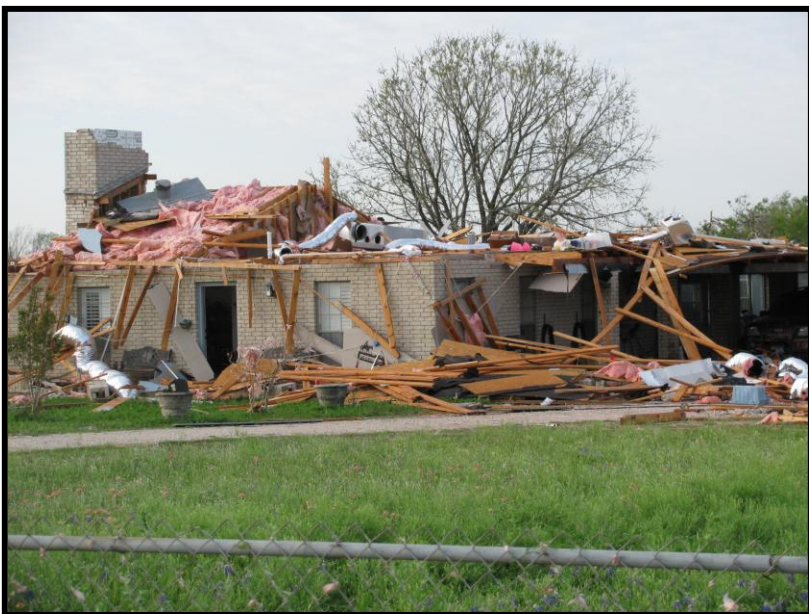
Figure 8. A home severely damaged By the EF2 Tornado in southwestern Bexar County, TX, on March 19, 2012.
