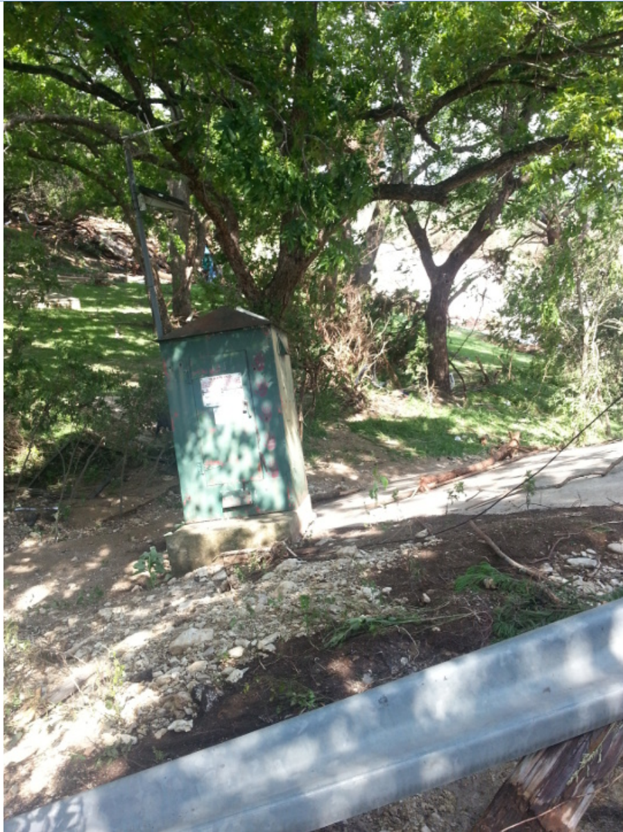
USGS Gage Housing at Ranch Road 12 Bridge (Blanco River at Wimberley, TX) on May 24, 2015.
