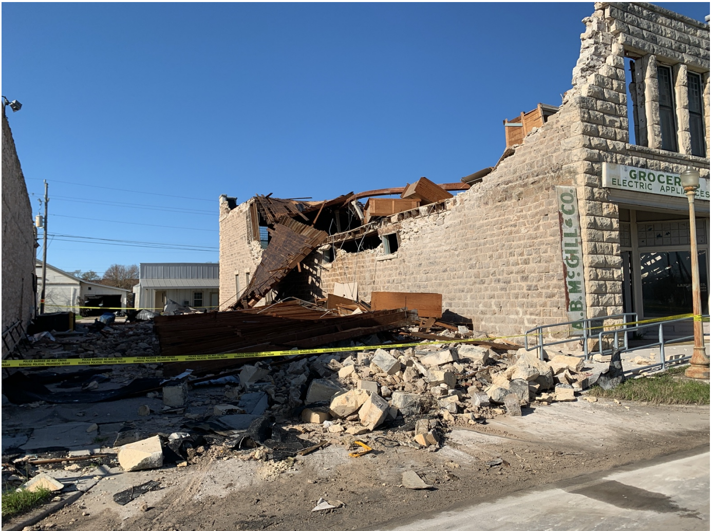
Straight-line wind damage in Bertram, TX
