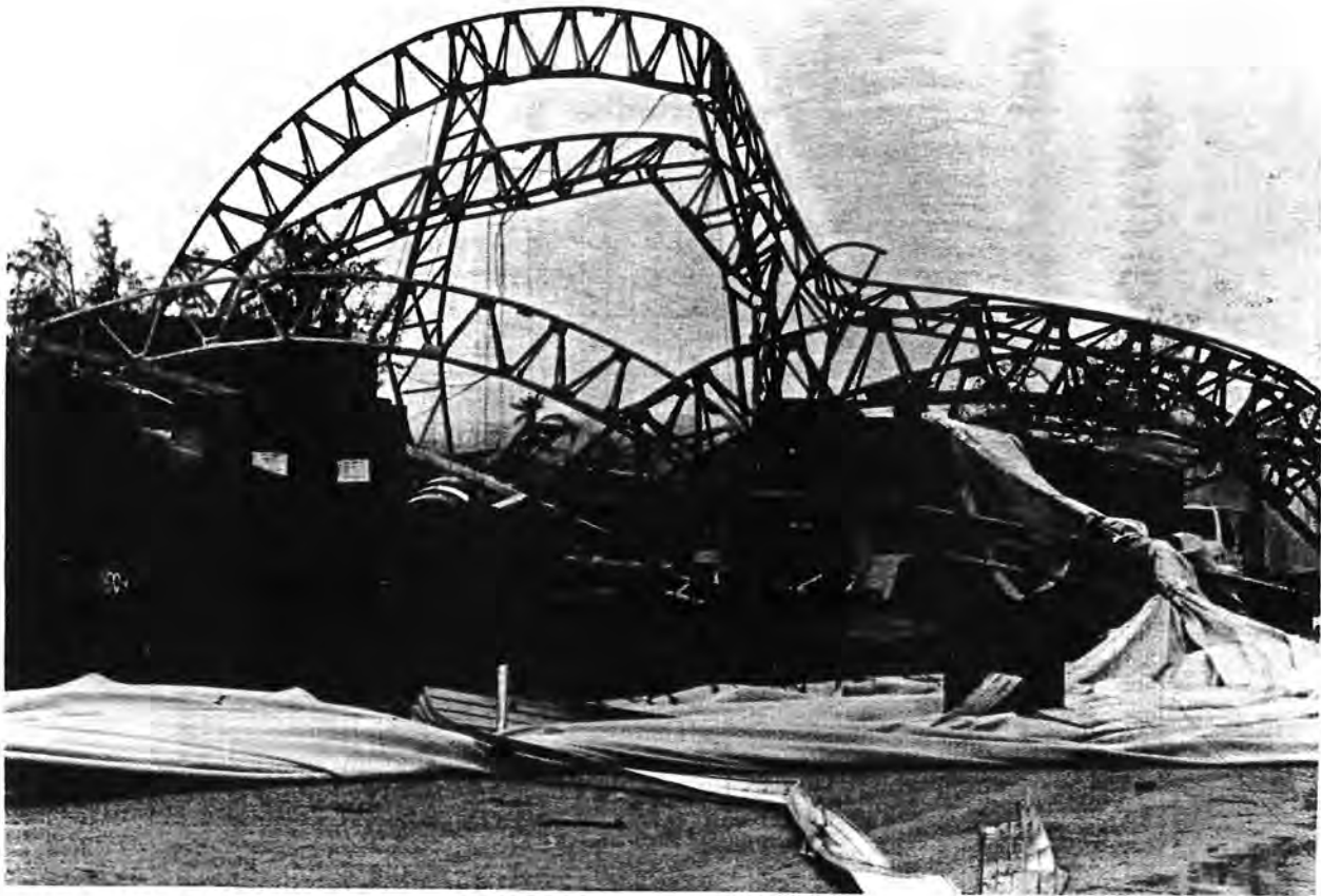
Figure 17. The steel girders of this temporary warehouse on Naval Station, Guam, were twisted by the high winds and collapsed during Russ's passage.
