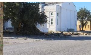
Wind damage to a church in Pecos, TX on Jan 21st
