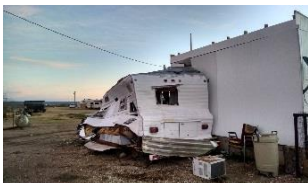
Wind damage to a mobile home in Pecos County on Jan 1st
