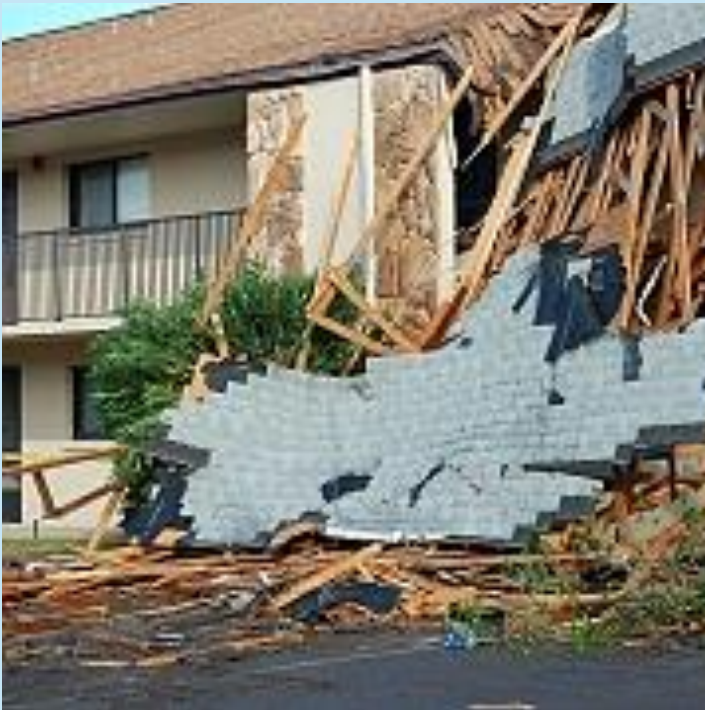
Part of the roof from Diplomat Condo where it landed on nearby Windrush Condo
