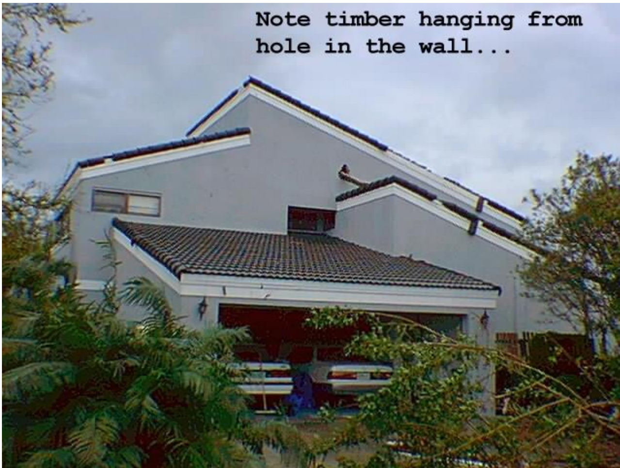
Damage photo at location 1.
