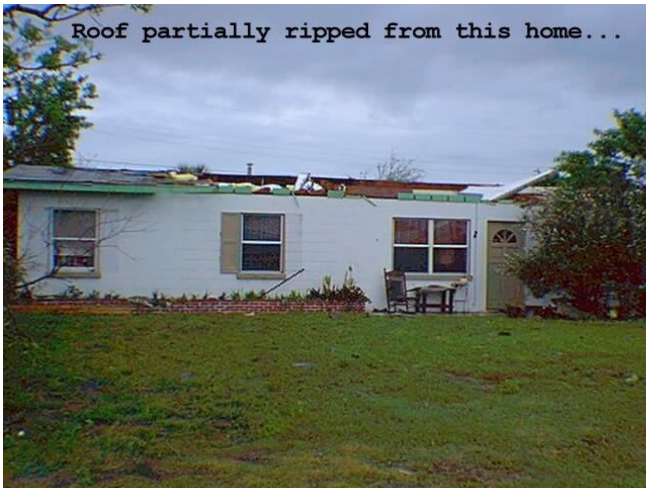
Damage photo at location 4.
