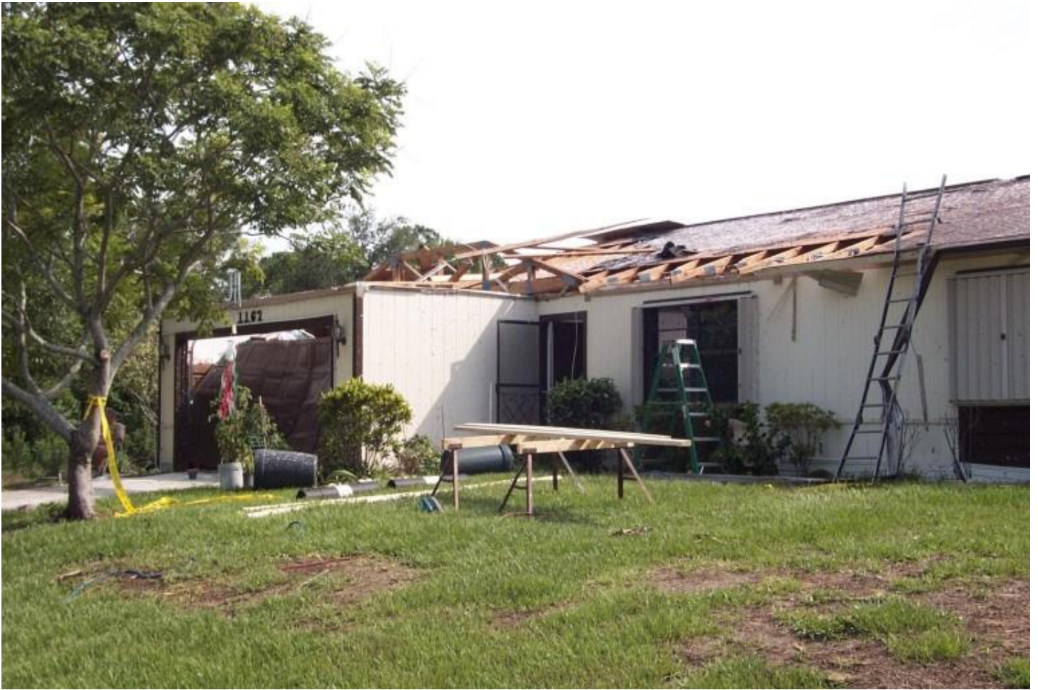
Significant roof damage (F1) to home.
