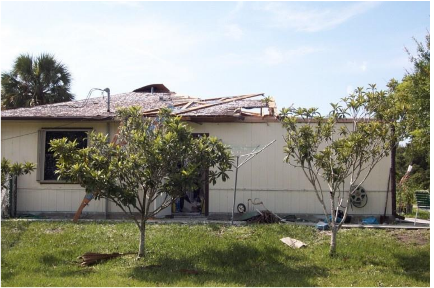
Different perspective of roof damage to same home.
