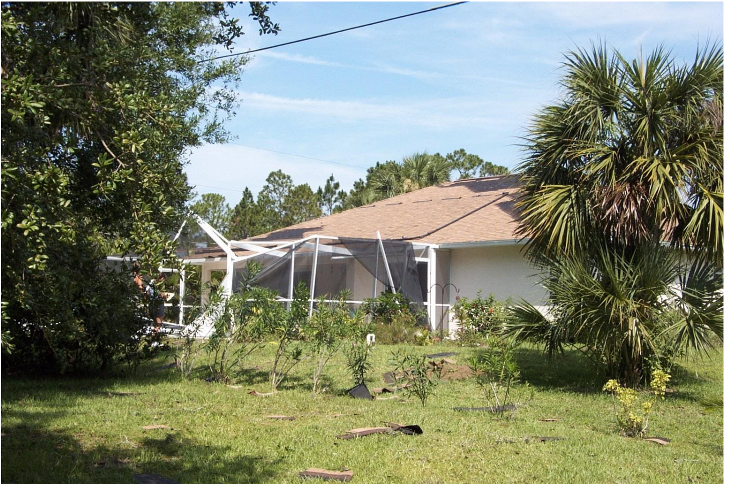
Pool enclosure destroyed and roof damaged.
