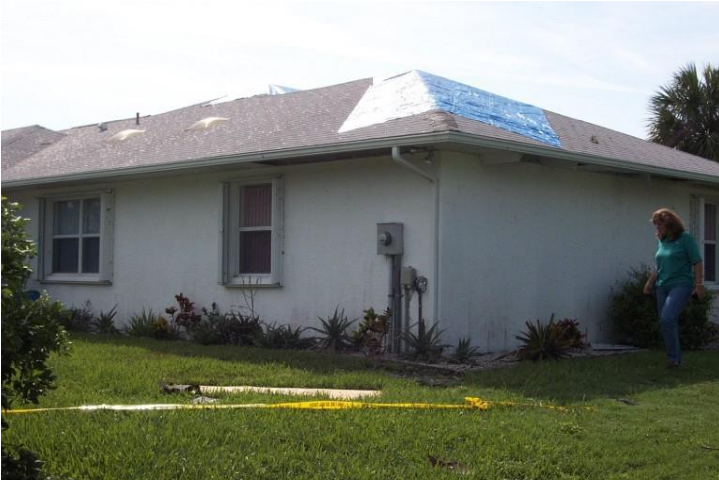
Roof damage to back of nearby home.
