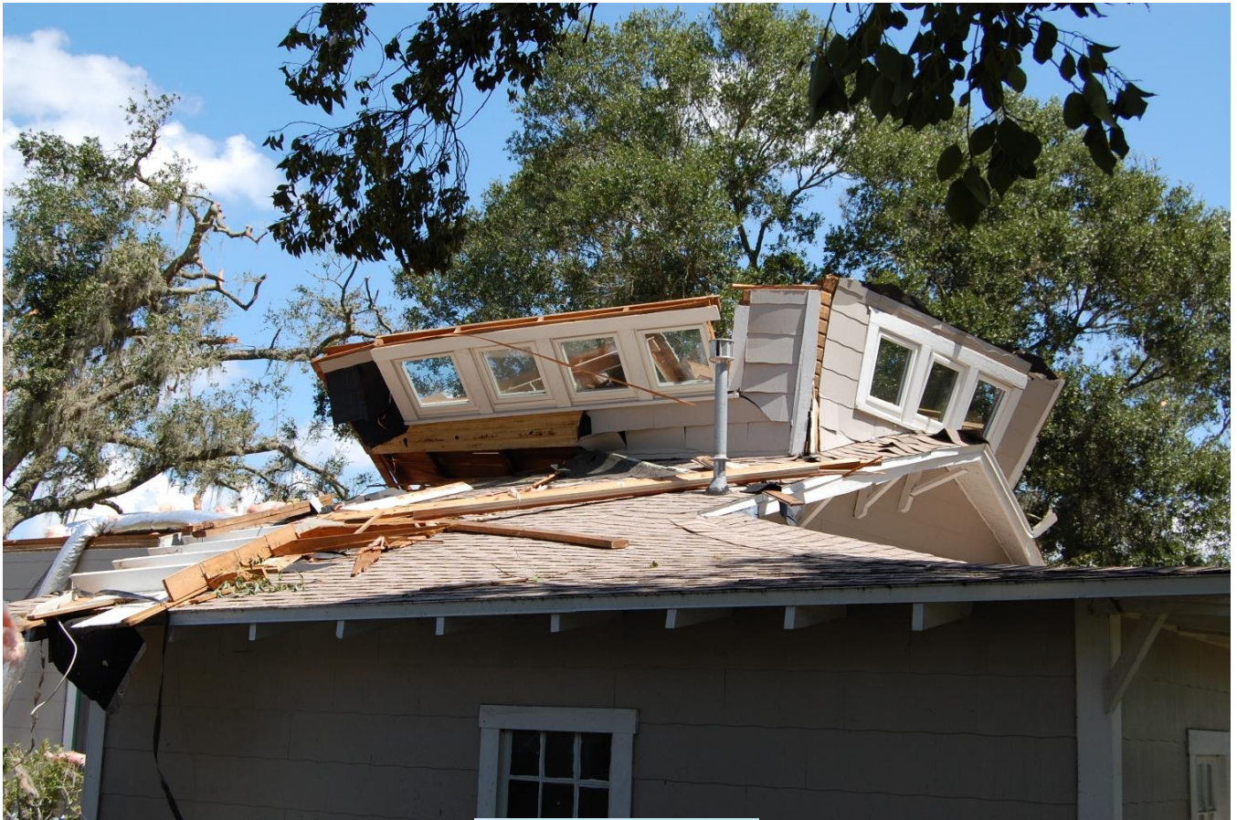
EF-1 Damage to Home
