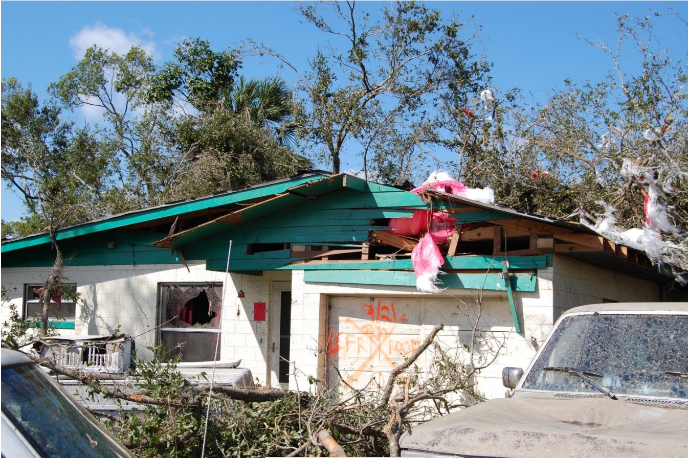
EF-1 Damage to Home
