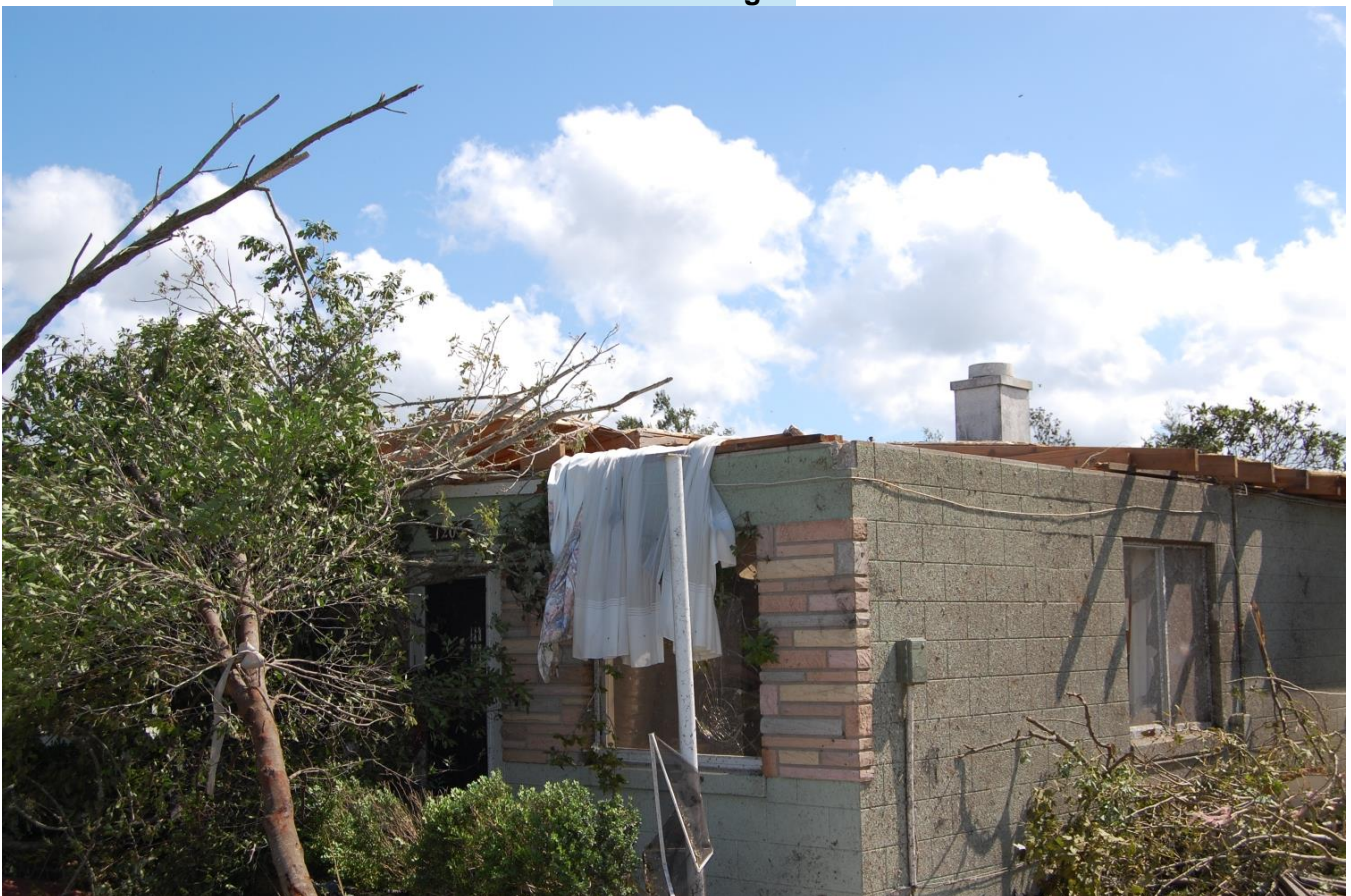
EF-1 Damage to Home
