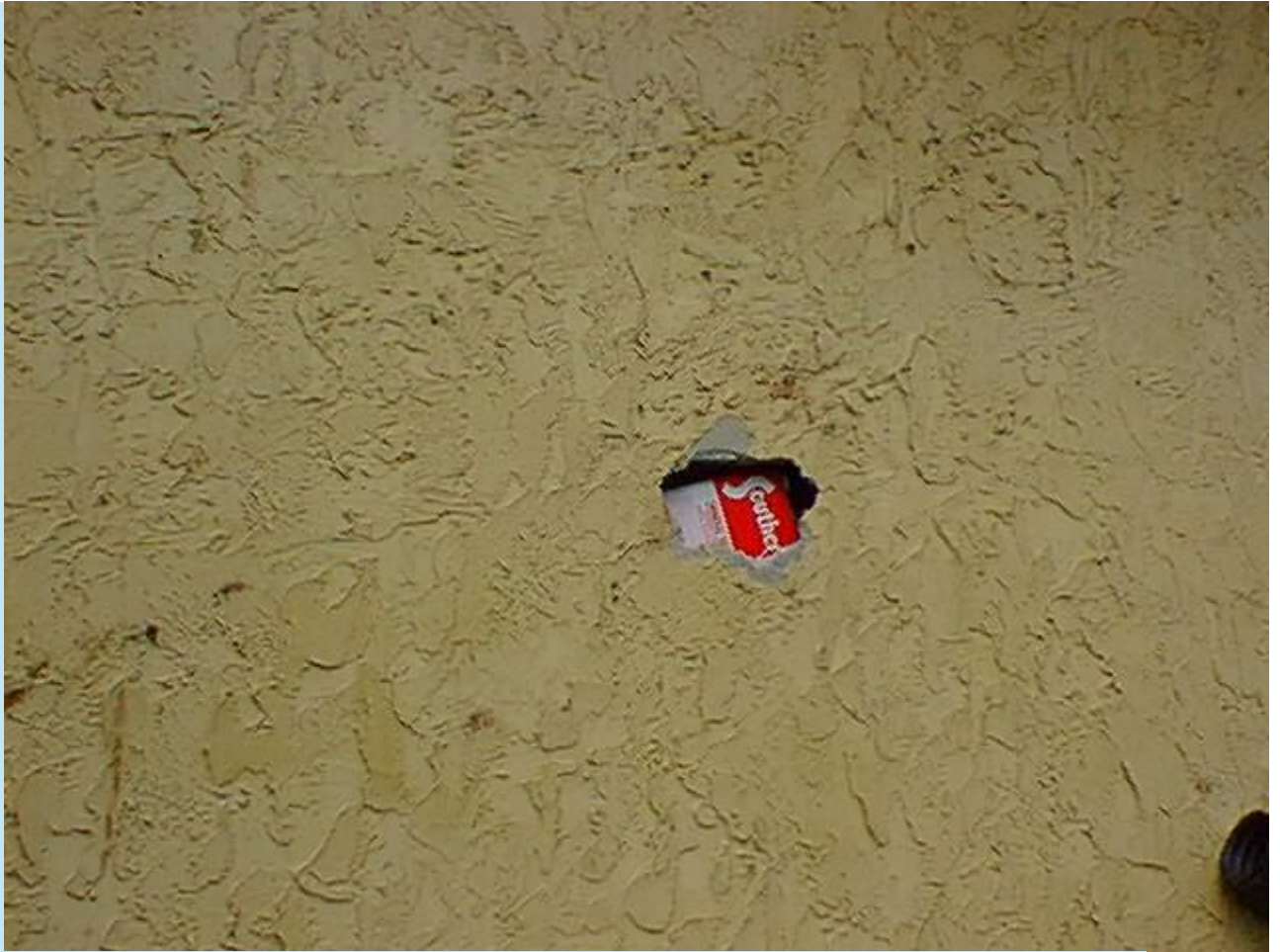
Hole knocked through block garage wall, Airpark Road
