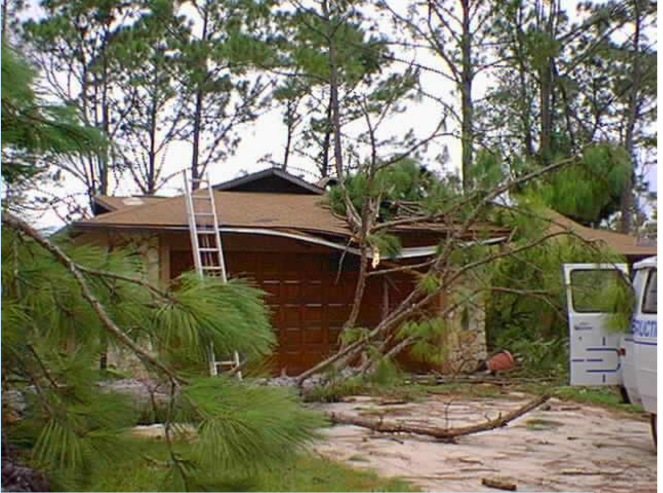
Tree damage to home
