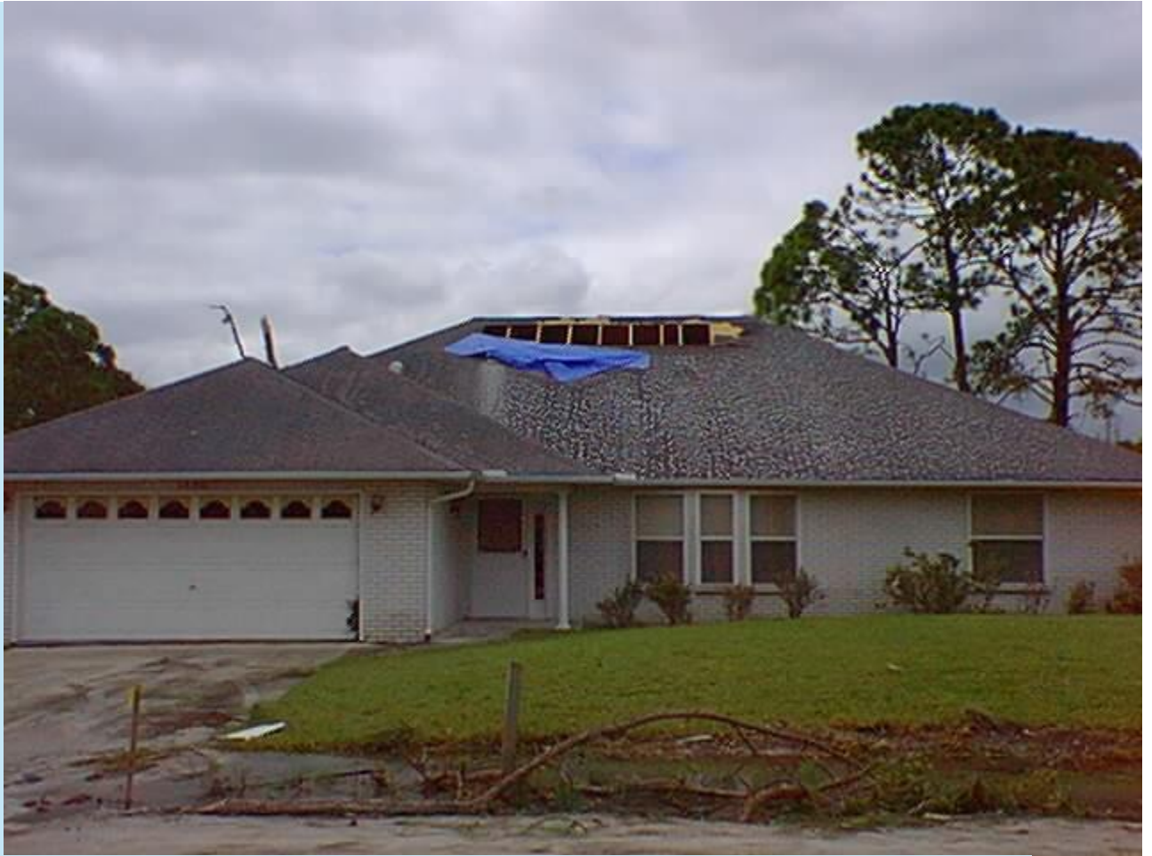
Severe Roof Damage
