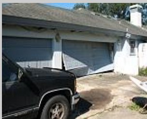
F0 damage to home in Seminole County
