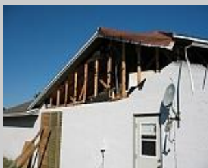
F0 damage to home in Seminole County
