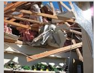
Damaged interior of home in Seminole County
