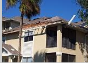
F0 damage to apartment building in Orange County.
