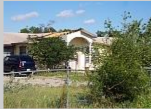
F0 damage to home in Orange County
