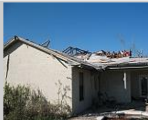
F1 damage to home in Seminole County
