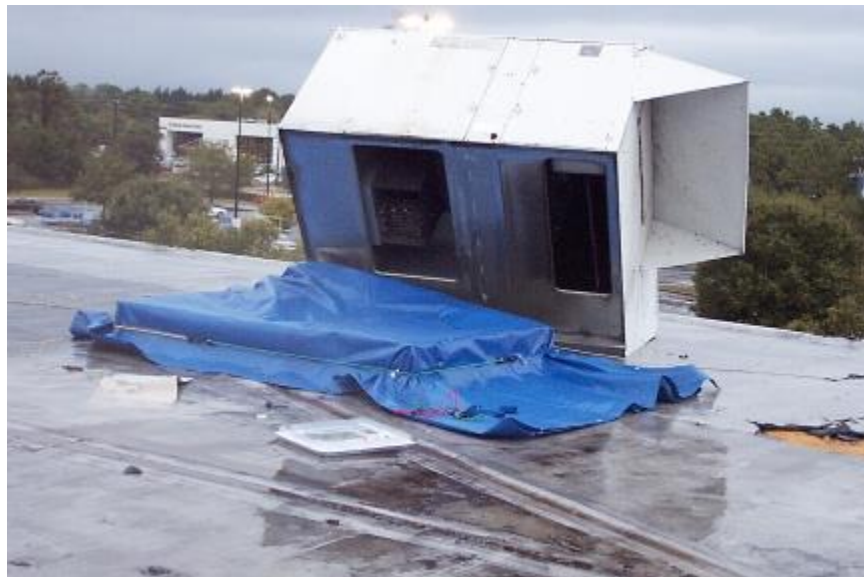
1800 pound air conditioning unity torn from roof
