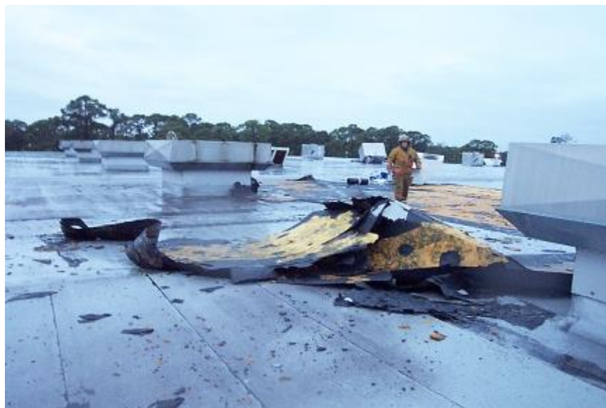
Roof damage to a building
