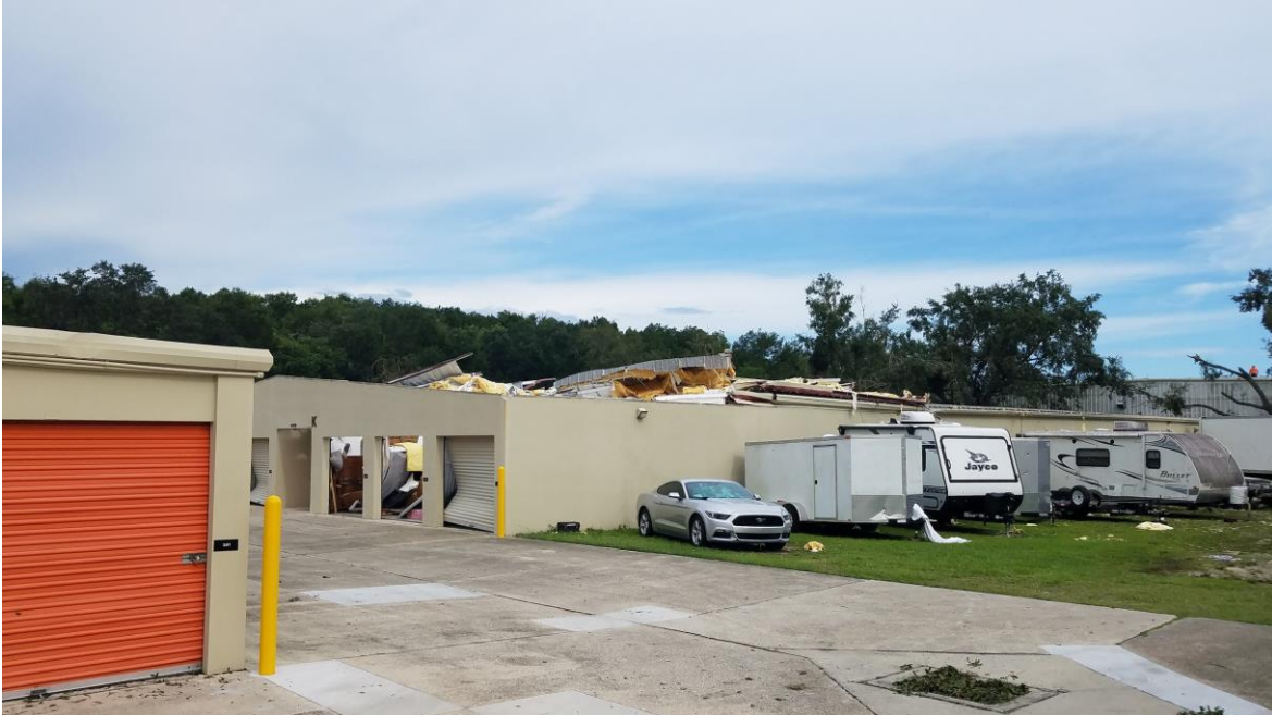
EF-1 damage occurred at a storage facility near W Plymouth Ave & Spring Gardner Ave
