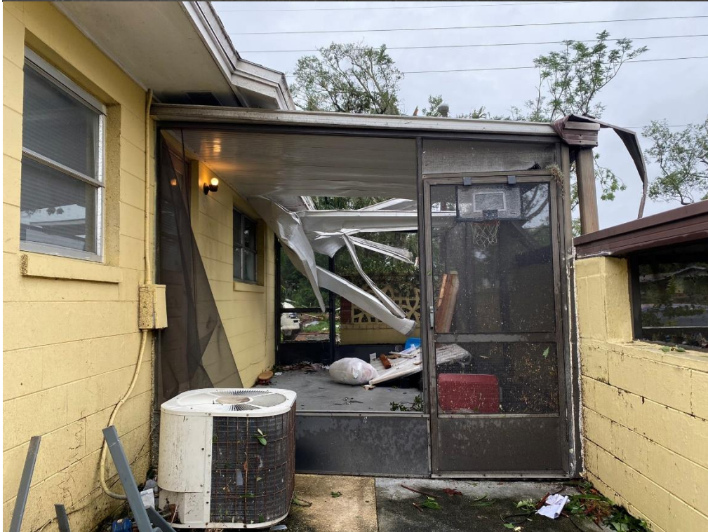
Worst damage at the Lake Margaret Village Apartments (both pictures) (peak winds estimated 100-105 mph, EF-1)
