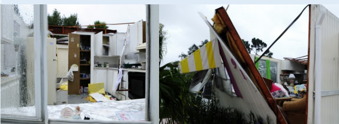
Damage to mobile homes from an EF-1 tornado in Barefoot Bay
