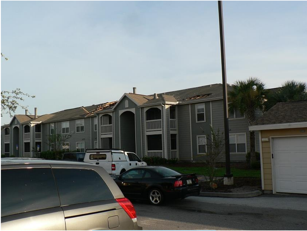
Tornado Damage in West Melbourne
