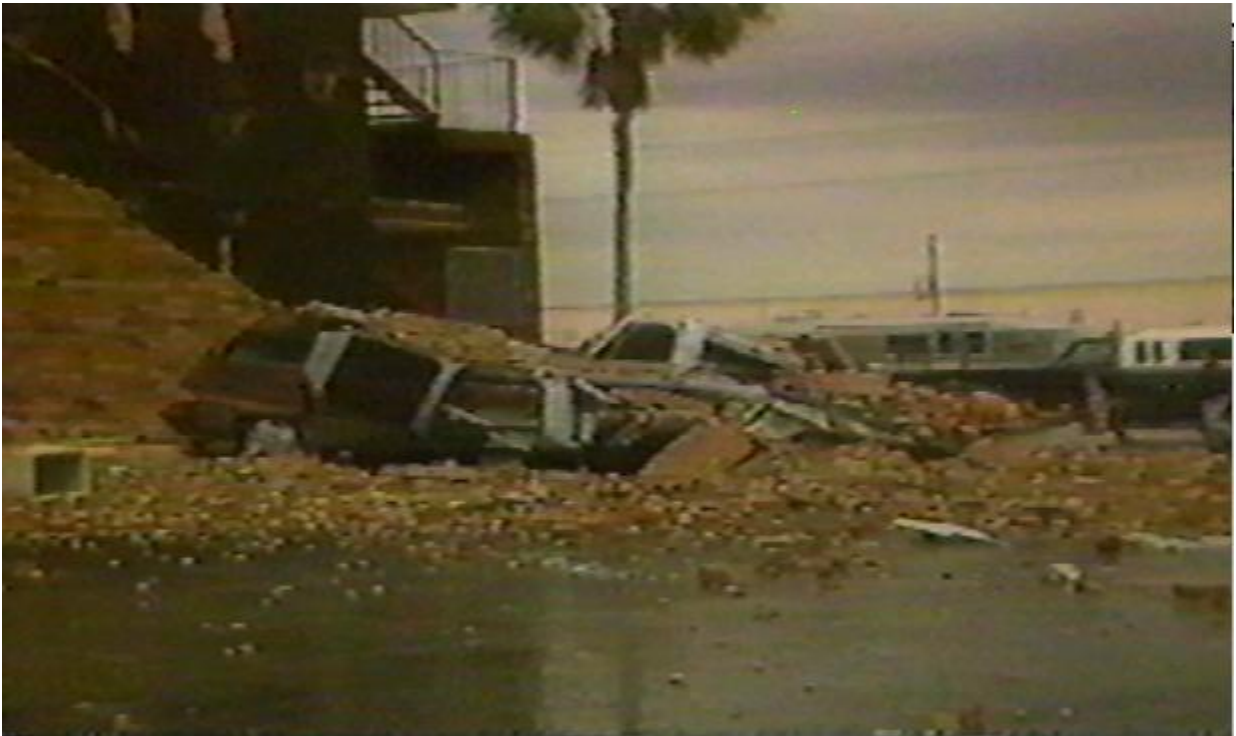
Severe thunderstorm winds knock down hotel wall on parked cars.
