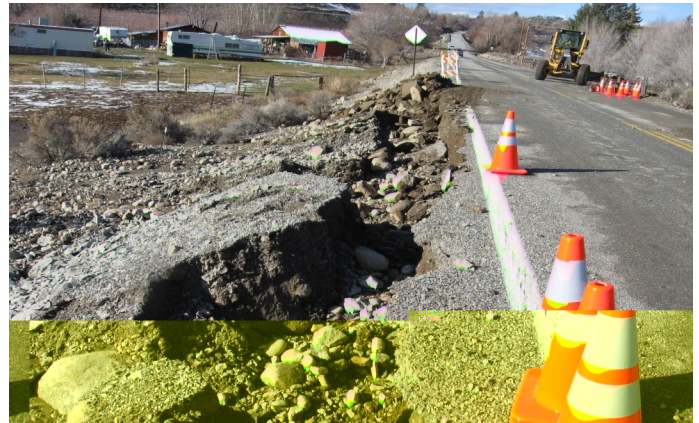
Winter water damage to portions of Highway 20 near Okanogan.
