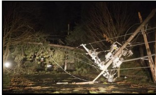
A familiar sight in Spokane, 11/17/15—downed trees and power lines on city streets
