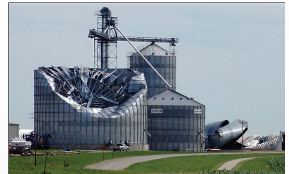
After a tornado, watch out for dangerous debris, such as sharp metal, glass, or downed power lines. Photo: NOAA
