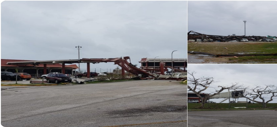
Pic. 1: Saipan's airport and a collapsed structure near the airport
