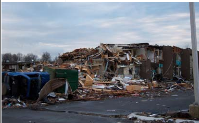
Damage from an EF-4 tornado which hit Union University in Jackson, TN. There were no fatalities and only minor injuries due to timely warnings from the NWS and proactive preparedness actions by the university. Photo courtesy of the NWS office in Memphis, TN.
