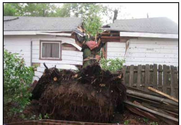
Split level anyone? Severe weather caused this destruction to a Battle Creek, MI, home.
