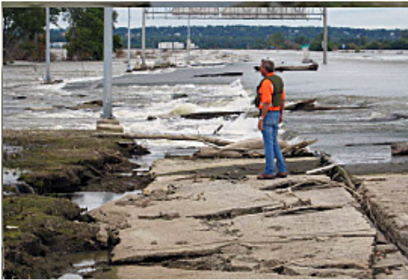
Damage to Interstate Highway 680 near Council Bluffs, IA. The Souris River crested in nearby Omaha, NE, at 36.29 feet on July 2, 2011, which was around 2 feet above the level shown on the photo dated August 16, 2011.
