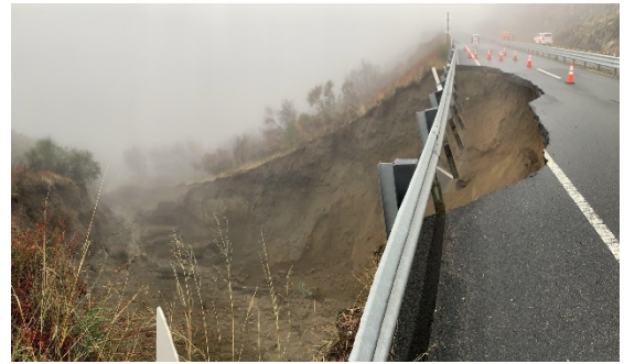
Damage to highway 18 from Christmas Eve's heavy rainfall.
