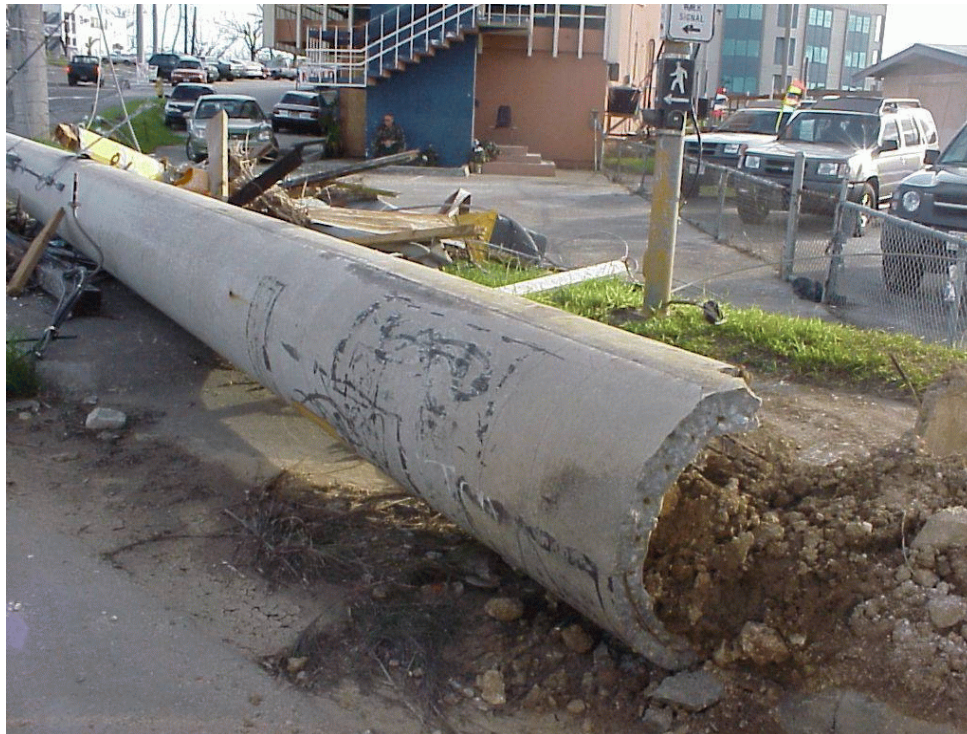
Downed utility pole along a back road east of the Bank of Guam (upper right) in Agana, Guam. (NOAA)
