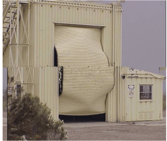
Picture 3. Severely damaged inflation shelter at Upper Air Facility. Courtesy of WFO San Diego.
