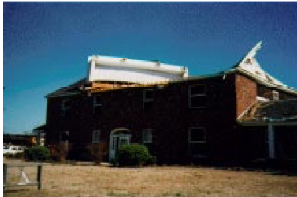
Photograph of brick church in Arkadelphia with major roof damage and broken windows. This church was on the edge of the downtown area where major destruction occurred. Courtesy of Chris Smith, NWS Southern Region.
