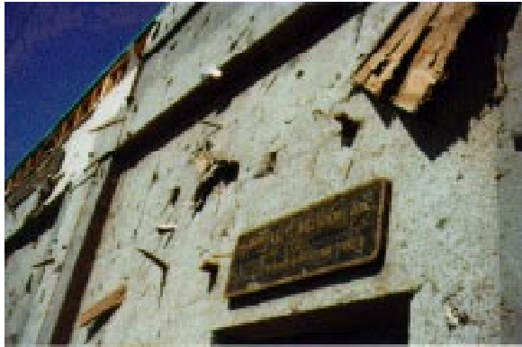
Photograph of old concrete and block building in downtown Arkadelphia where major destruction occurred. Flying debris knocked holes in the walls and wooden boards pierced the side of the building. Courtesy of Chris Smith, NWS Southern Region.
