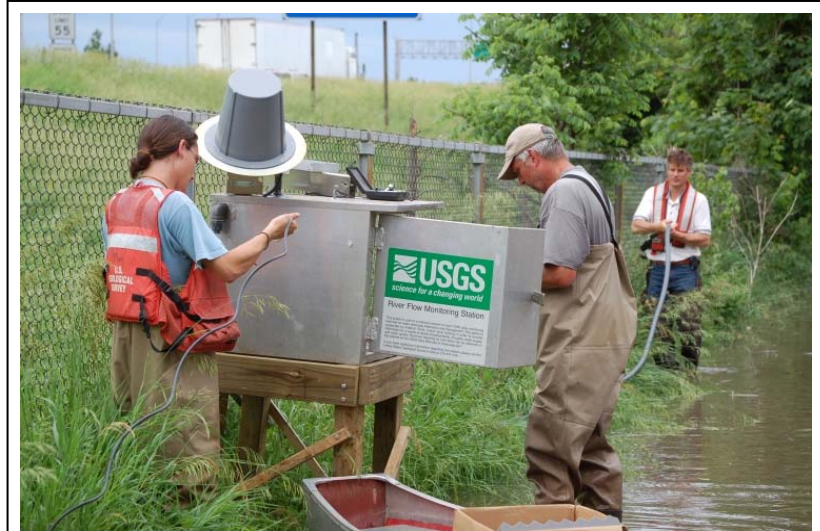
Fig. 18. USGS staff installing temporary streamgage at 13th Avenue and J Street in Cedar Rapids, Iowa, June 12, 2008. (USGS photograph by Don Becker.)
