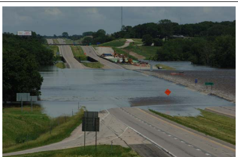
Fig. 10. Cedar River overtopping Interstate 80 in eastern Iowa, June 13, 2008 (looking east). (Used with permission. ©2008 Iowa Department of Transportation. Photograph by Kevin Arrowsmith.)
