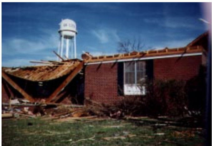
Damaged home, Vista Ridge subdivision, Van Buren
