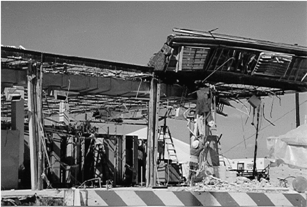
Damage to a telephone switching station caused by the Pedernales Valley tornado. Photograph by M. Trainor, NOAA.
