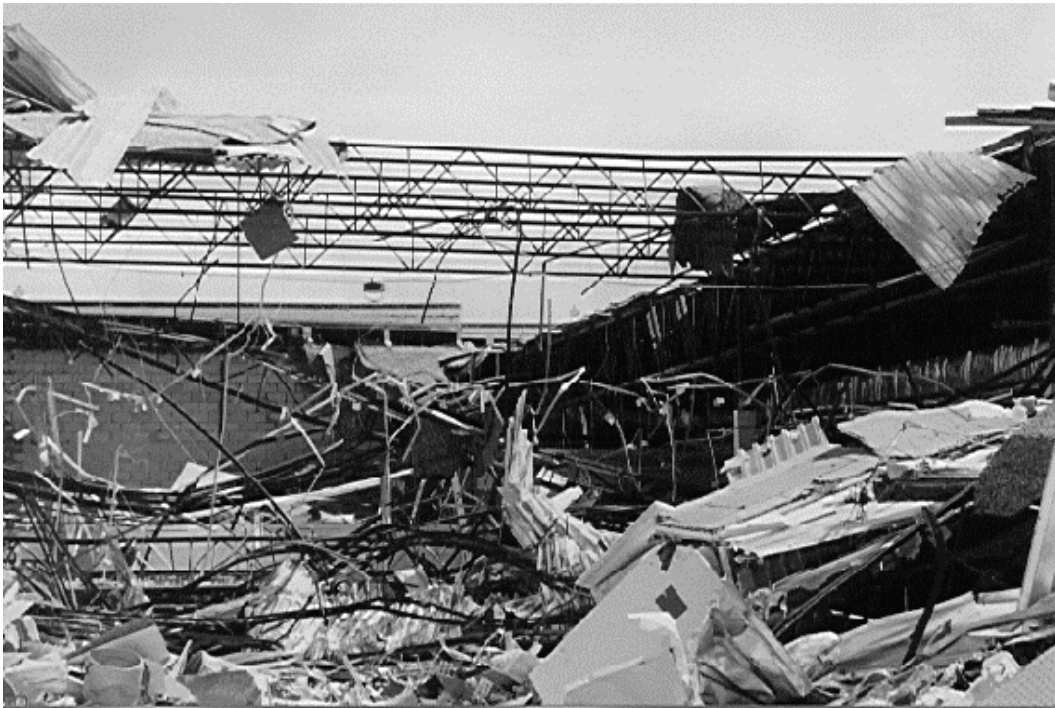
Ground view of damage to Albertsons grocery store. Photograph by M. Trainor, NOAA.
