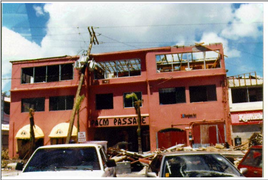
Figure 1-10. Damaged commercial building along the Charlotte Amalie Harbor. (Photo courtesy of Matt Stout)
