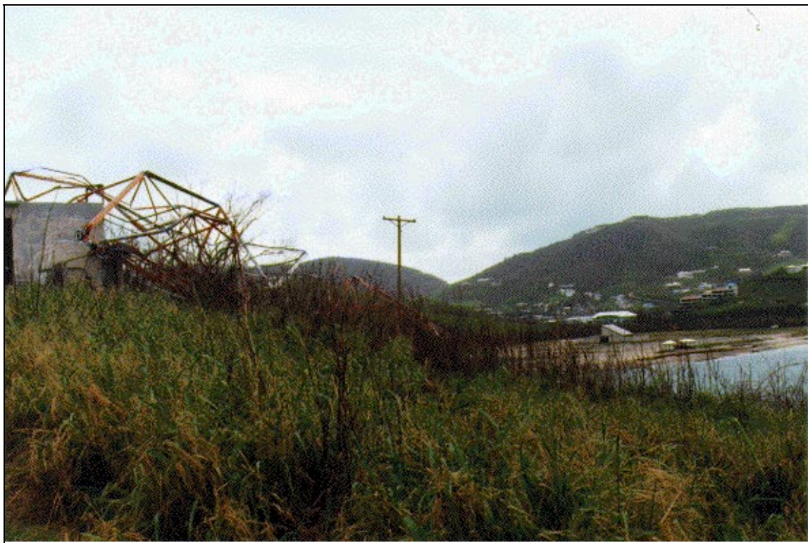
Figure 4-1. WSTX radio's tower collapsed during Marilyn. (Photo courtesy of Matt Stout)
