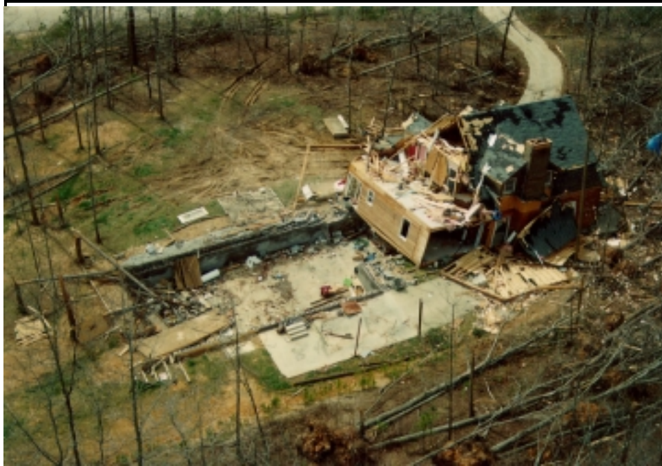
Unanchored home shifted off its foundation. Most of the home, including the garage, moved to the north (Calhoun County, Alabama). Photograph courtesy of _____.
