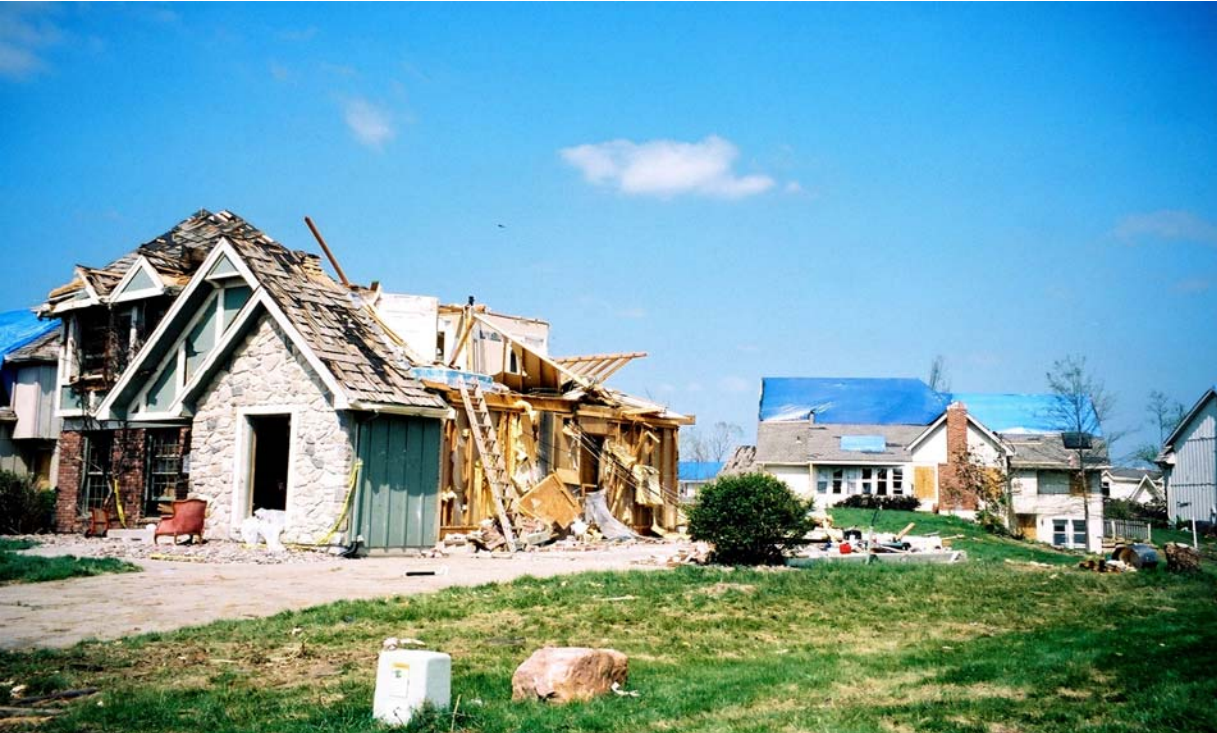
This housing subdivision in north Kansas City suffered major damage on May 4.
