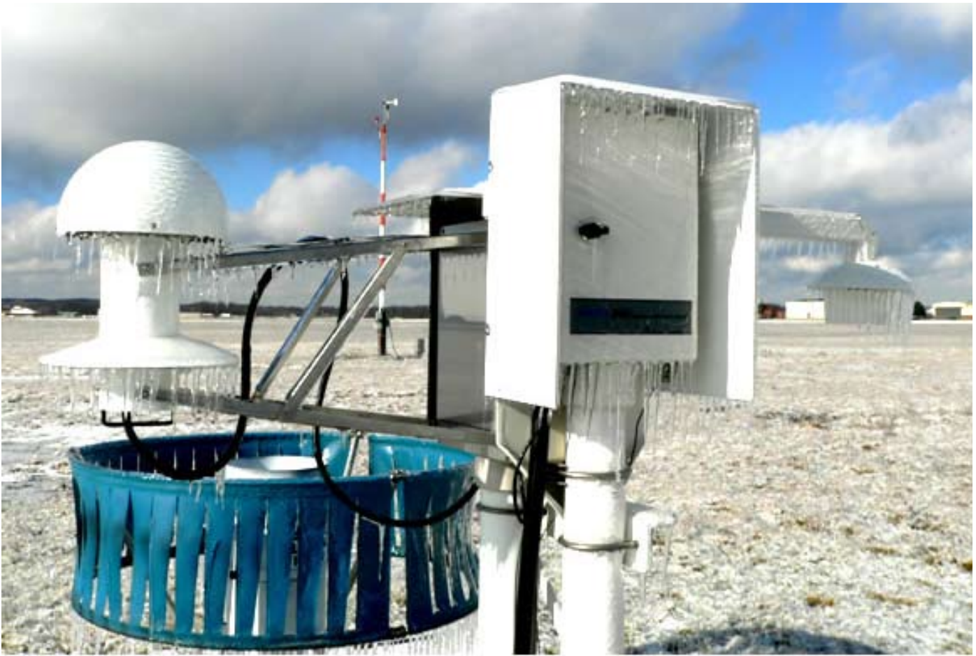
Shown above are a frozen temperature sensor, dewpoint sensor and heated tipping bucket on an ASOS unit. In the past, during periods of icing or freezing precipitation an entire array of ASOS weather equipment could freeze up or malfunction. ASOS now includes an Ice Free Wind Sensor as well as improved freezing rain sensors. Photo by NWS Grand Rapids, MI, Electronics Technicians Eric Repaal and Thomas Williams.
