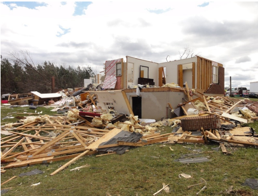
Fig. 7a. Damage to a home just south of Evergreen, VA near the start of the tornado track.
