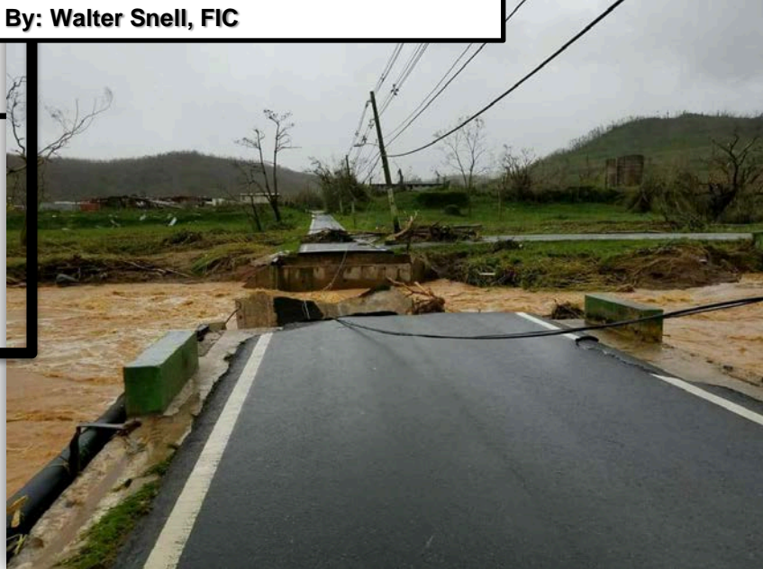
Figure 1 The bridge over the Canóvanas River looking east up highway 957. The river had risen around 5 feet above the roadway at the height of the flooding. It likely failed after its central support had been undermined.
