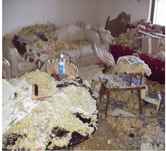
Insulation blown into home after roof damage in Manatee County
