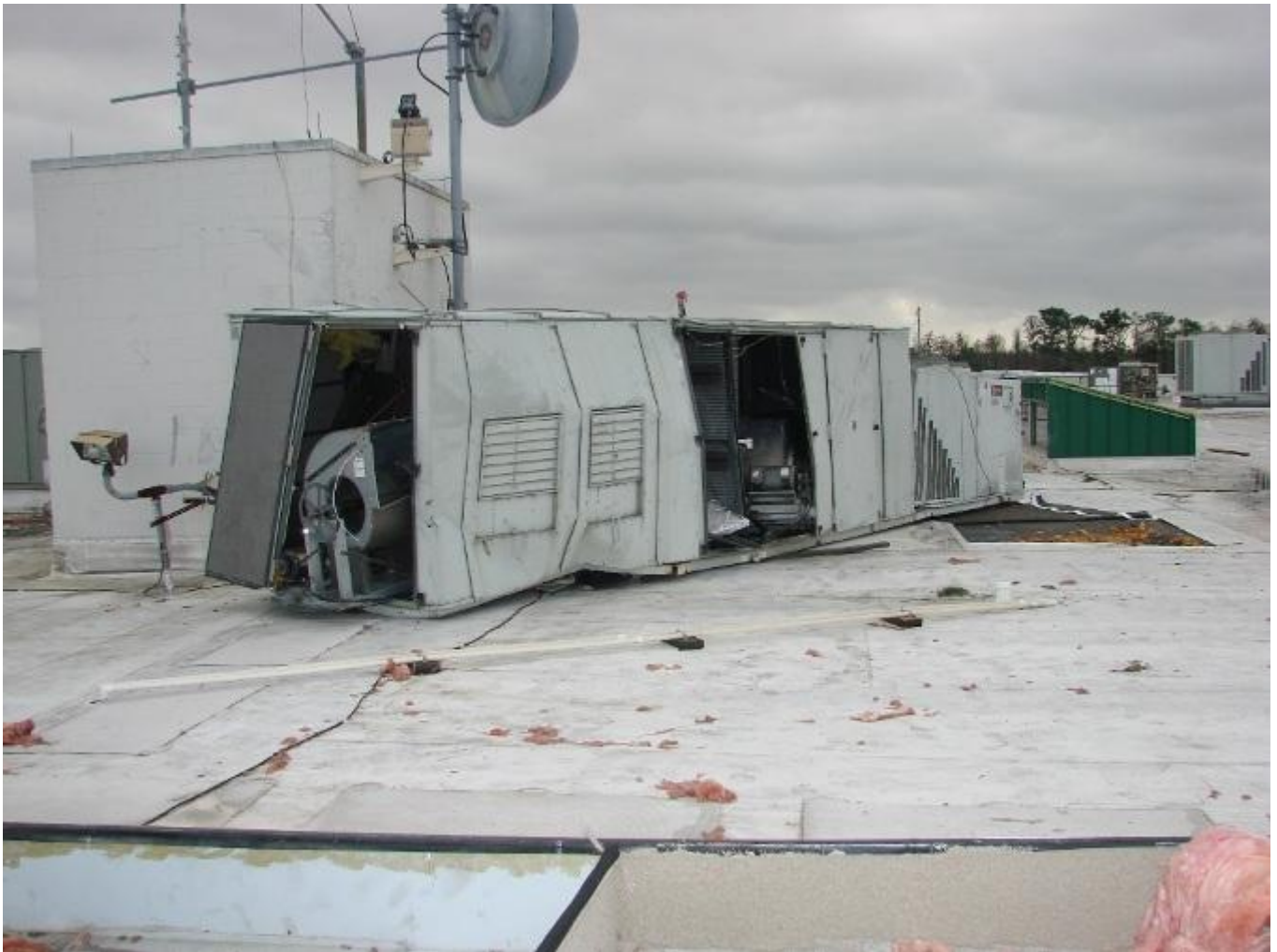
Figure 5. Site C damage (Jailhouse air conditioning roof units).
