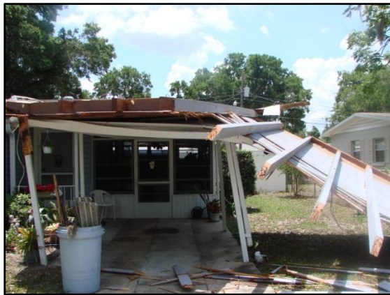
A piece of the dislodged carport rests on a structure
