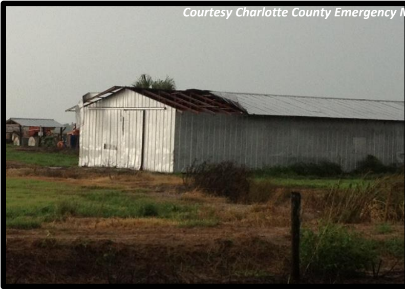
Wind damage to roof of metal outbuilding. Courtesy of Charlotte County Sheriff's Office
