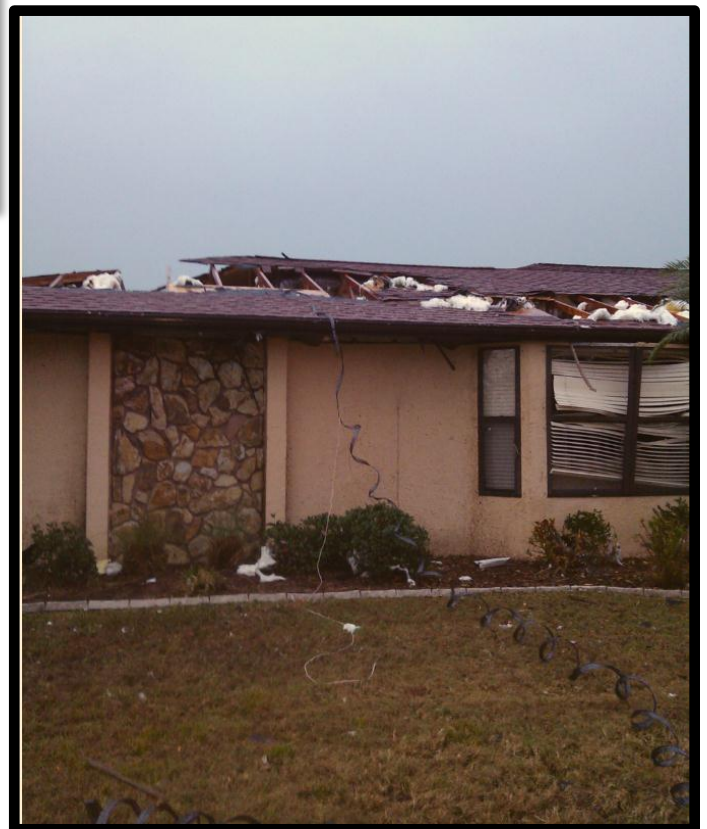
Tornado Damage at Point 2. Courtesy of Charlotte Co. EM
