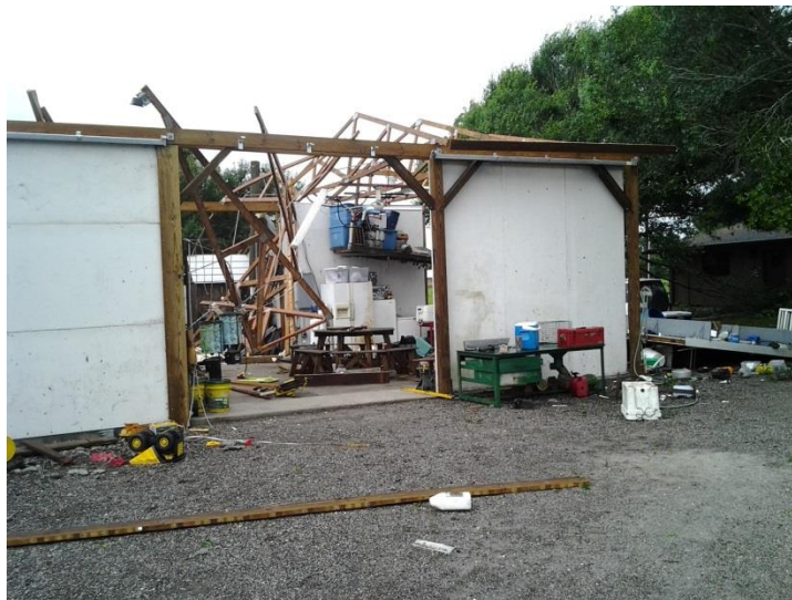
Myakka City tornado damage.
