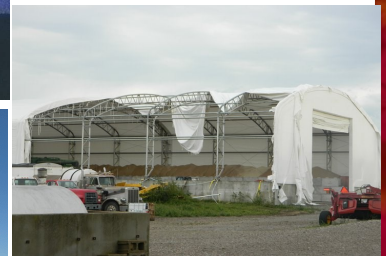
This outbuilding near Whiting, KS was destroyed by the August 19m wind storm. Photo courtesy of Luca Cochren
